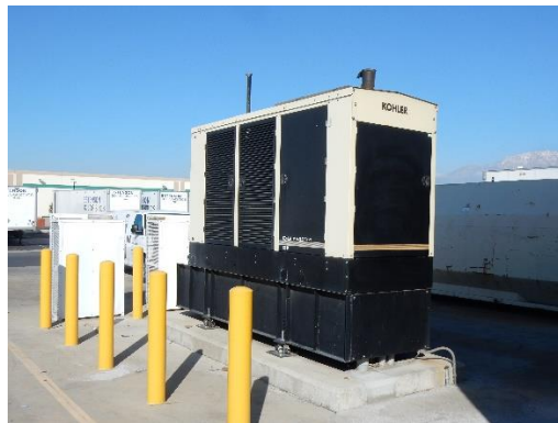
Figure 10 Confirm all Enclosure Doors are Closed and Latched
