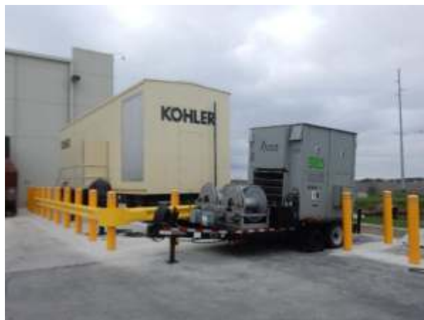
Figure 2 Confirm all Enclosure Doors are Closed and Latched
