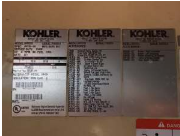
Figure 1 Make, Model and Serial Number Tag on Generator
